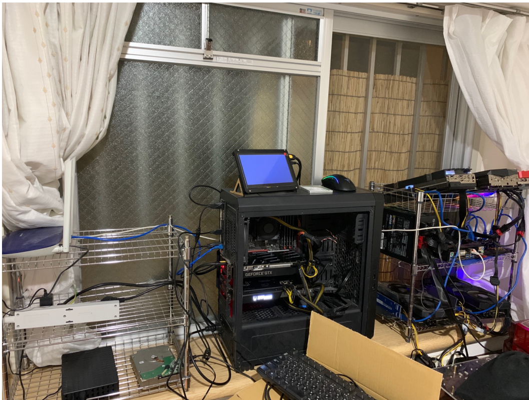
Figure 3. Liang's Ethereum mining rigs are positioned beside his bedroom window to have better ventilation. 15
